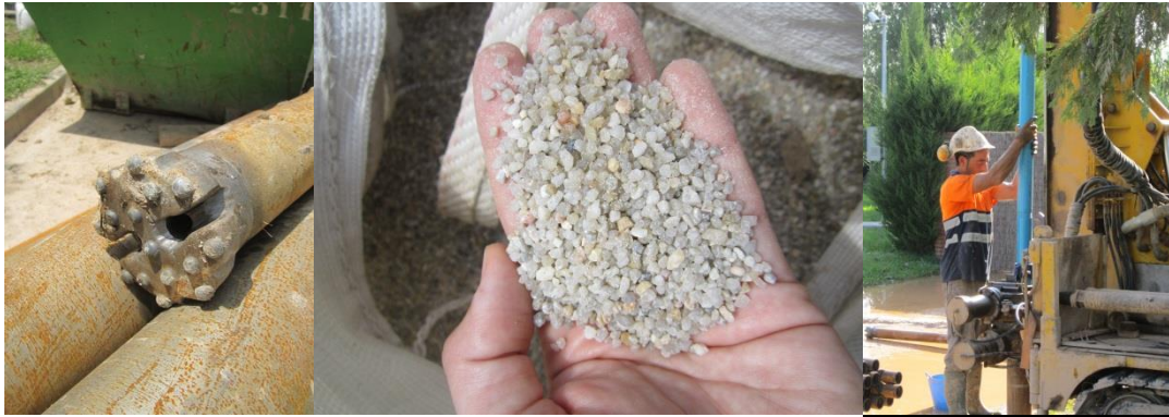
Figure 11: Drilling works of Pz2 in Sant Joan Despí (See in the middle details of pre-filter material)
